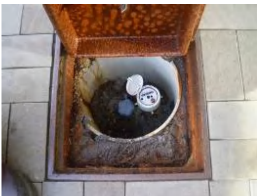
Figure 3-6 : Commercial water meter installed on Camp Street
