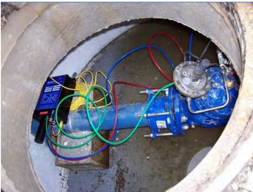
Figure 3-4 – Flow modulated PRV on Windsor drive
