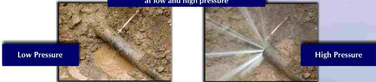
Figure 5: Typical burst water main at low and high pressure
